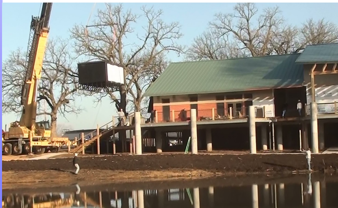
In 2012 Seeser Crane carefully slides the 8,000 gallon, 18-foot long, aquarium into the Eco Tourism Center.
